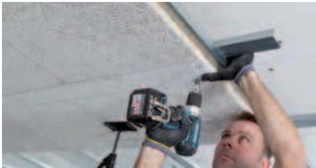
Install the acoustic tiles with the aid of a support. When fixing, press the tile onto the profile using the heel of your hand. There must be no gap between the tile and the profile. Begin tile installation from the centre of the room. Only handle the acoustic tiles with clean hands (clean gloves are recommended) and clean tools.
